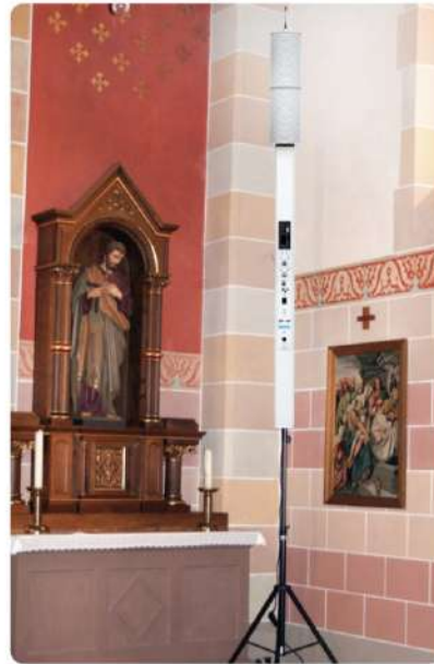
Fig.: above ZP-SLIM as a stationary sound system in the church
